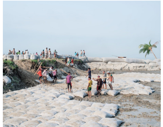
Sandbags being laid for the foundation of a river bank defence, at Elisha Ferry Ghat, on the bank of the Meghna river on Bhola Island, Bangladesh where as much as 18% of the countries land mass could be inundated by sea level rise.
